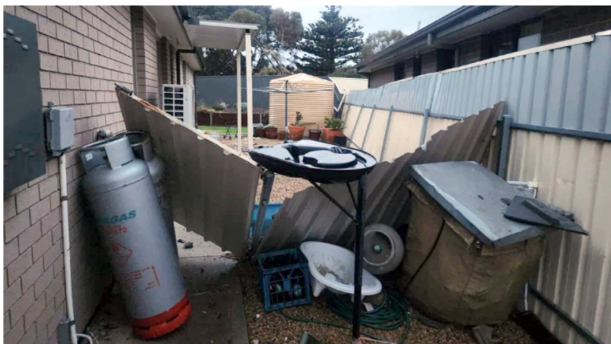
Storm damage to a side gate which in turn knocked 2 x 45kg cylinders off balance causing considerable strain on the high-pressure pigtail connections.
