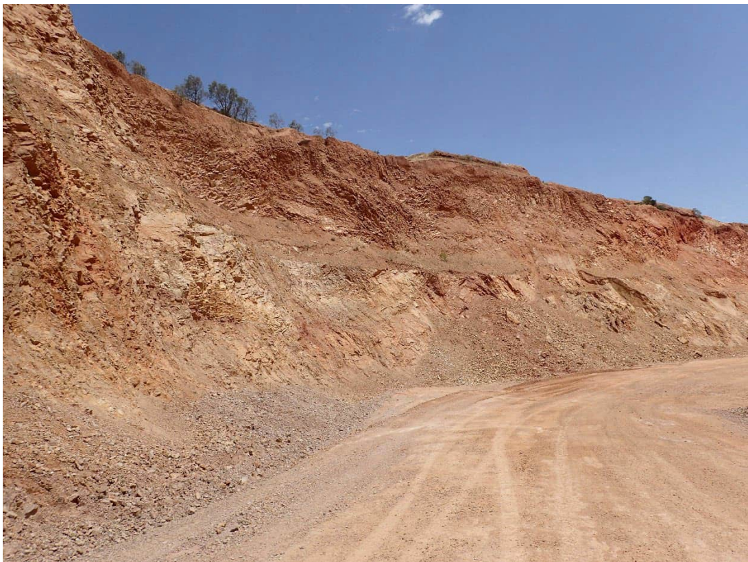
Figure 4: Image displaying the jointed and broken nature of the highwall rock mass.
