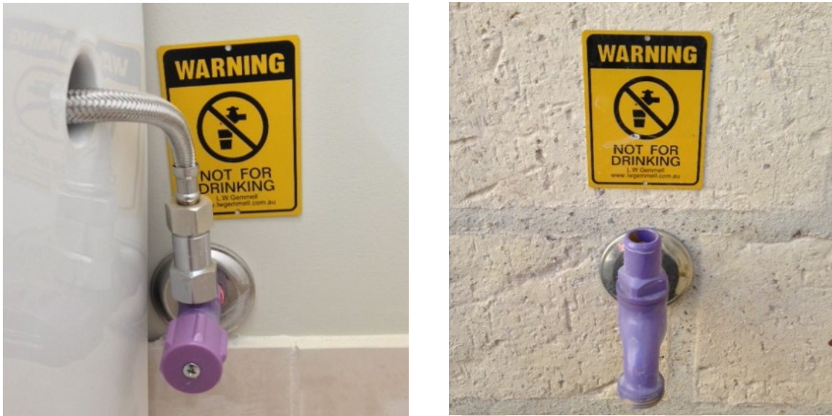
Figure 2-3 Examples of non-drinking water plumbing signage
