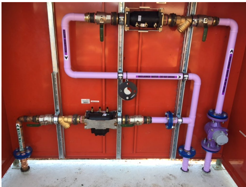
Figure 2-5 Reduced pressure zone valves installation – Typical connection manifold to non-drinking water supply
