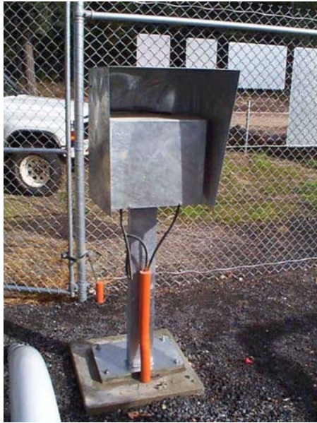
Lightening Protection Nangwarry.
