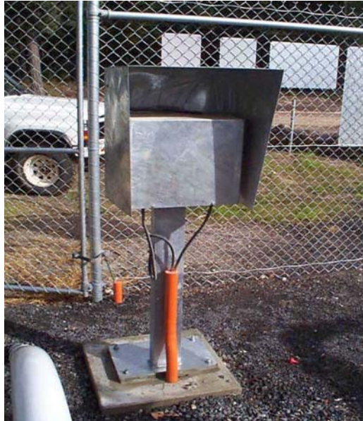
Lightening Protection Nangwarry
