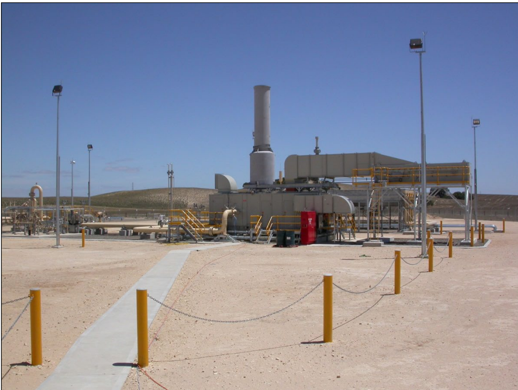
Plate 3-4: Coomandook Compressor Station
