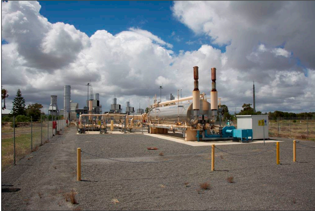
Plate 3-3: Quarantine Meter Station
