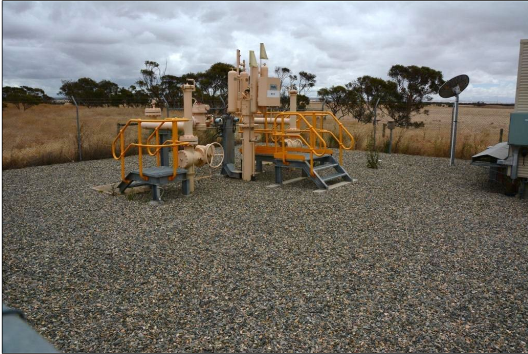
Plate 3-1: Pallamana Mainline Valve
