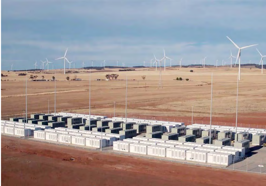
Plate 3 – Typical 150MW BESS, Hornsdale SA (Image supplied: Neoen Australia Pty Ltd 2017)
