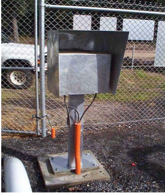
Lightening Protection Nangwarry
